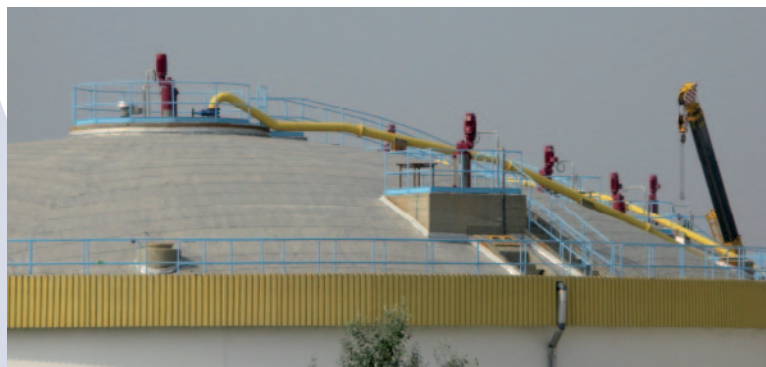
Digestion tank (with several agitators) - Baraki - Algeria
