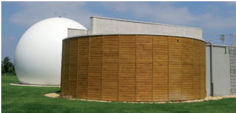
Installation for methanization of waste water plant sludge
